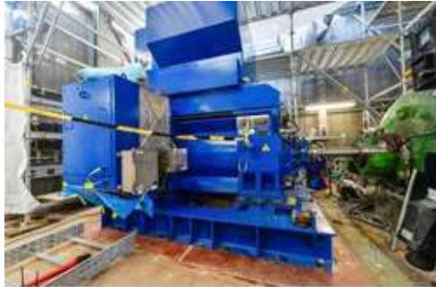
Fig. 21. Motor (L) - Compressor (R) after replacement
