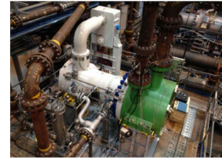
Fig.13 Single-Stage Motor-Compressor during string test
