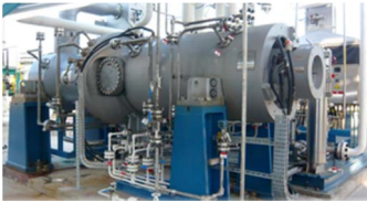
Fig.32 Ethylene Integrated Compression 2.8MW - 2.4kV - 11000 rpm 13 to 97 bars - 0.77 MSm 3 /day
