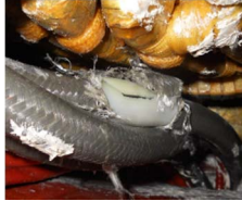
Fig.20 Cable Insulation Failure during Tests-3
