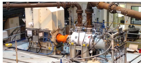
Fig.5 Standalone Motor Compressor during Shop Testing
