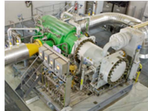
Fig.12 Pipeline Station 8.6MW - 6kV - 11000 rpm
