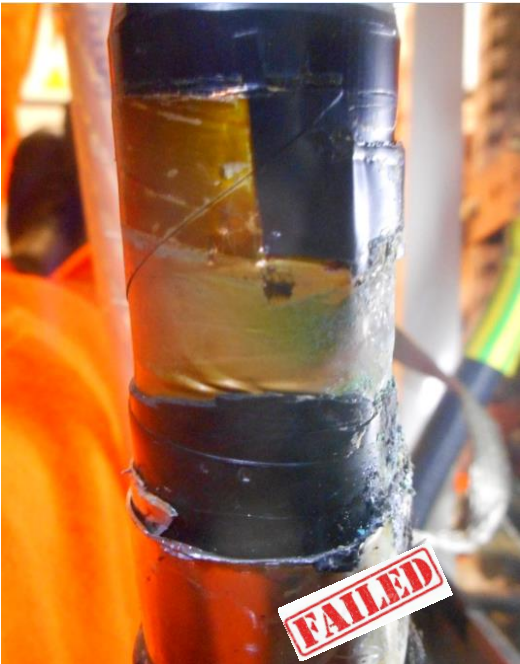
Poor contact between the cable screen and the ground braid due to a PVC tape forgotten
