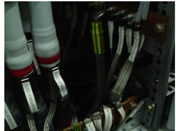
All shield not properly installed
