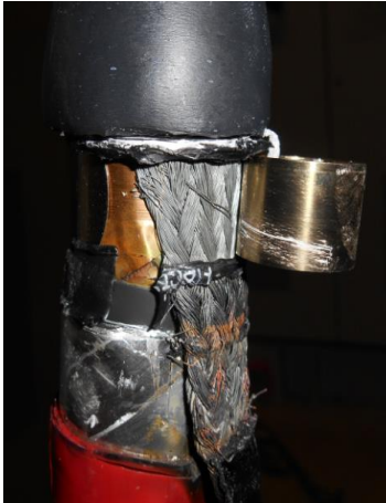
Earth braid onto the springs
