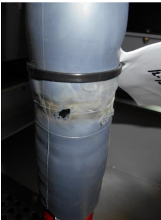
External failure mark
