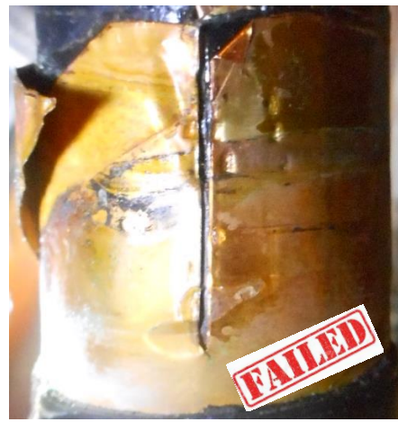
The cable screen has been cut without reason. The effect is to increase the contact resistance, thus overheating.
