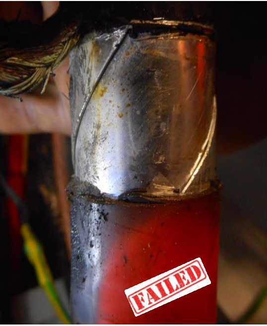
Poor contact between the cable armor and the ground braid due to the important thickness of the aluminum alloy tapes material.
