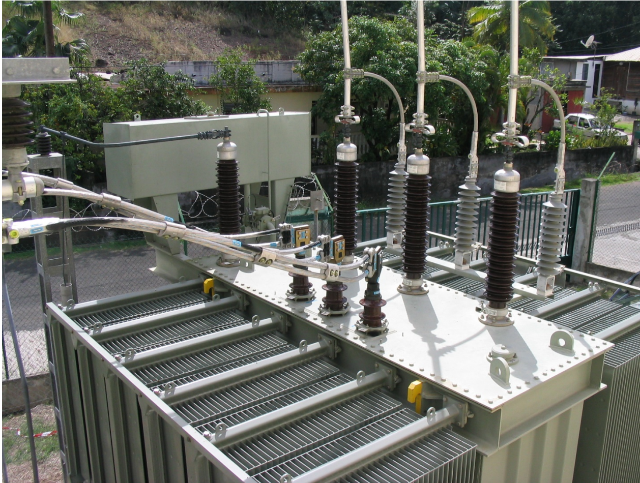
Arrestors located very close to terminals
