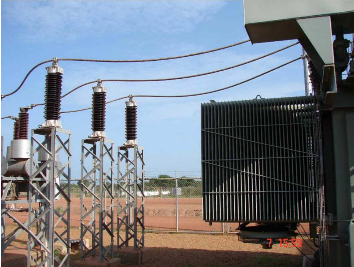
Arrestors located close to terminals on separate supports
