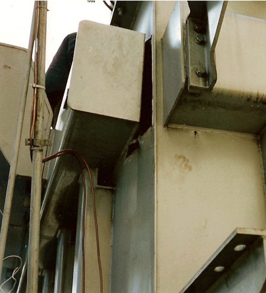
Tank ripped open in several locations
