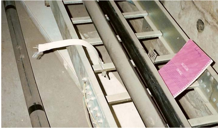
110 kV cable clamps broken
