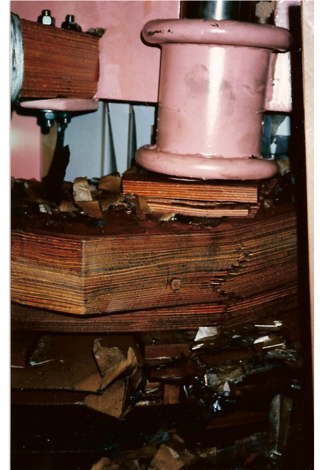
Extensive internal damage
