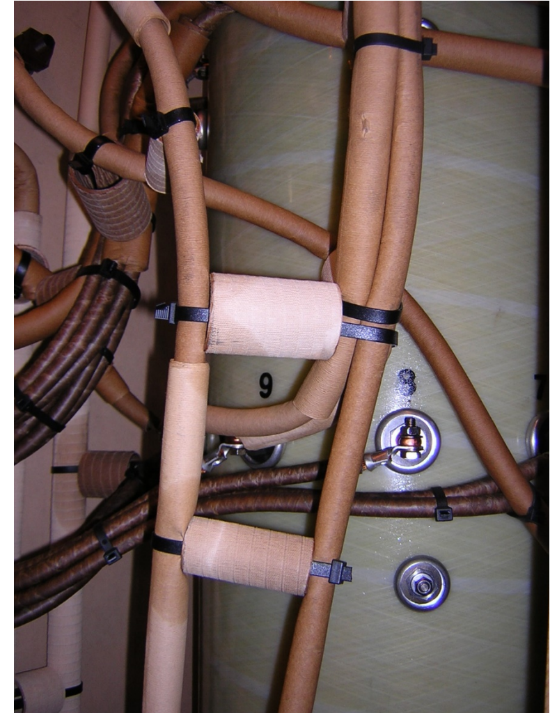
Increased separation distance after second repair
